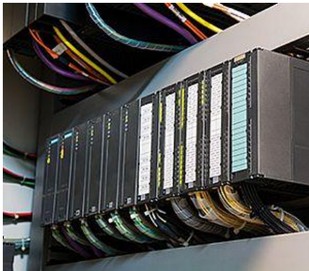
Programming Siemens PLC S7-1200
